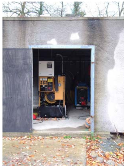
Figure 11 Generator awaiting access to the electricity grid at Camphill Community Ballytobin.
