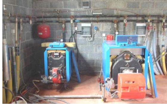
Figure 13 Two of the gas boilers, and part of the community heating system.
